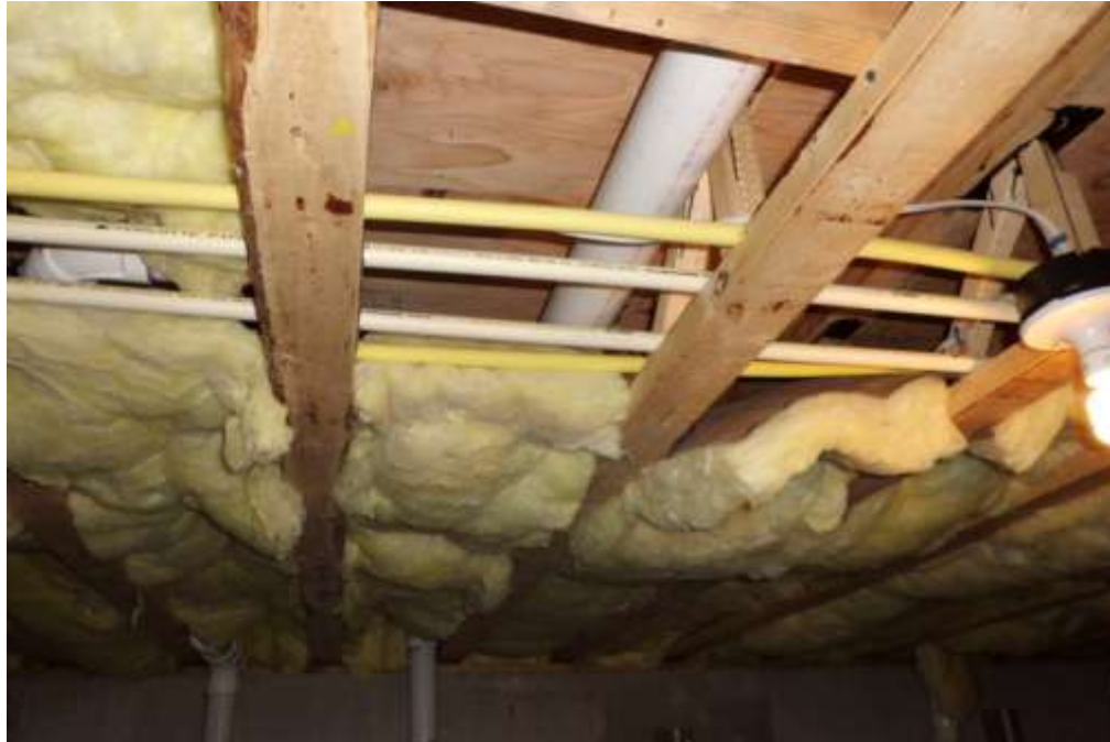
Figure E-5: Poorly Installed Frame Floor Insulation
