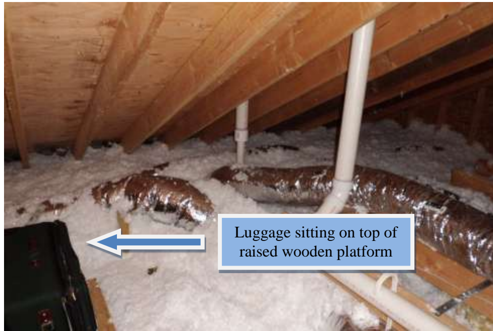
Figure E-11: Blown-in Fiberglass Attic Insulation with Storage Platform
