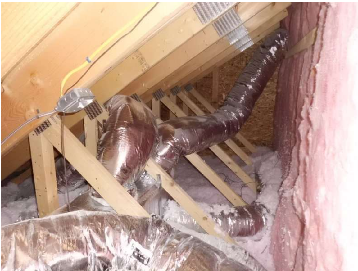
Figure E-14: Kinked Ducts Exposed to Wind-Washing Behind Knee Wall
