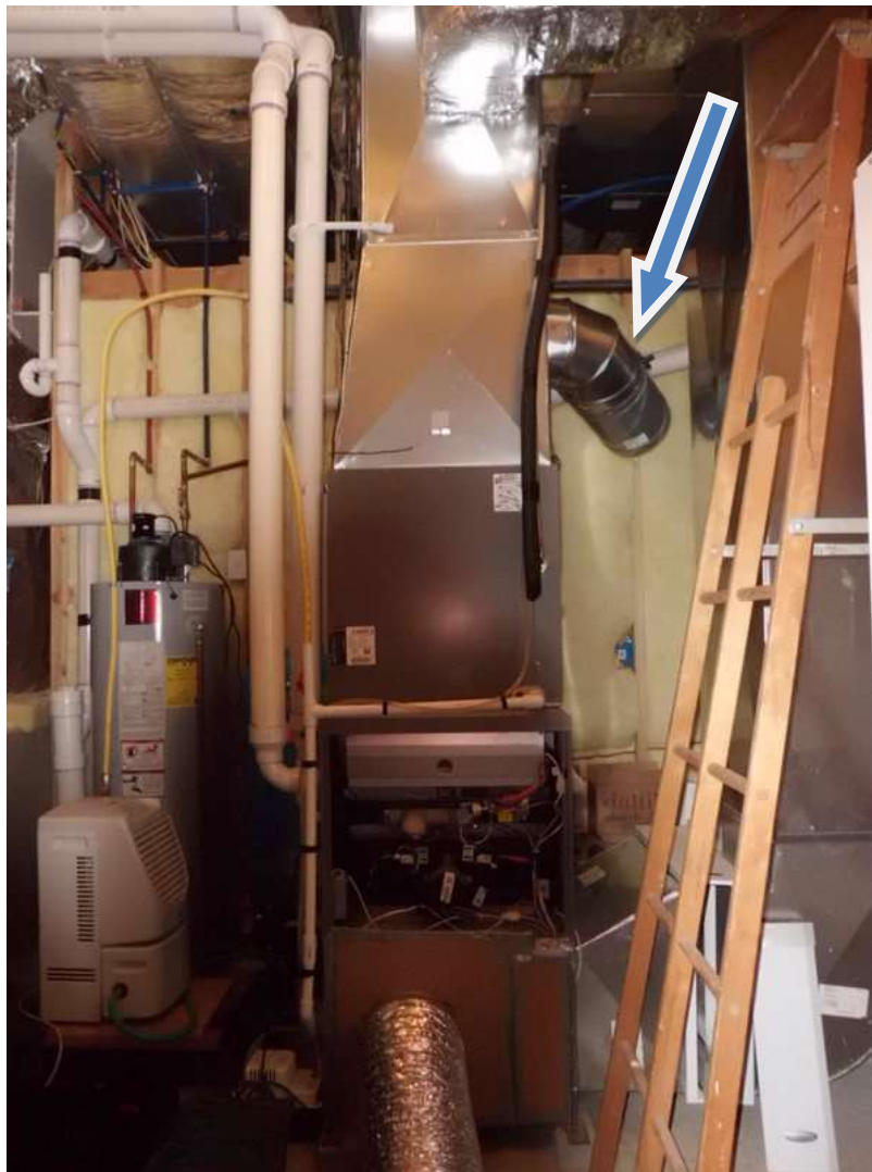
Figure E-16: Pressure Relief Diverter & Uninsulated Supply and Return Ducts
