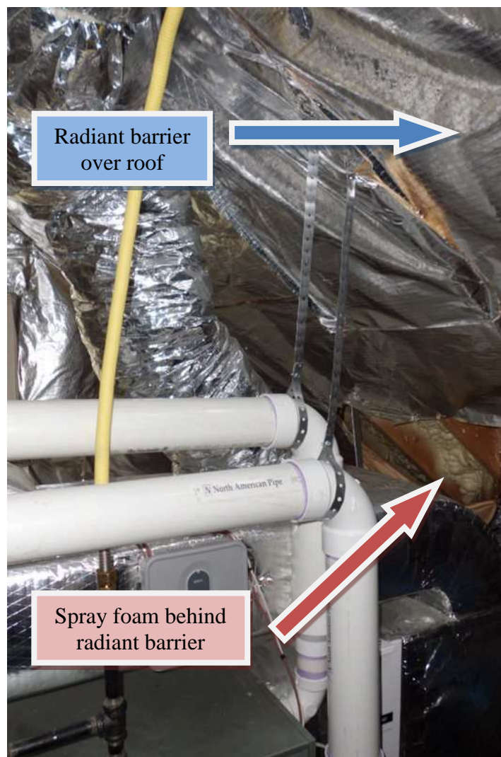
Figure E-13: HVAC System in Conditioned Attic
