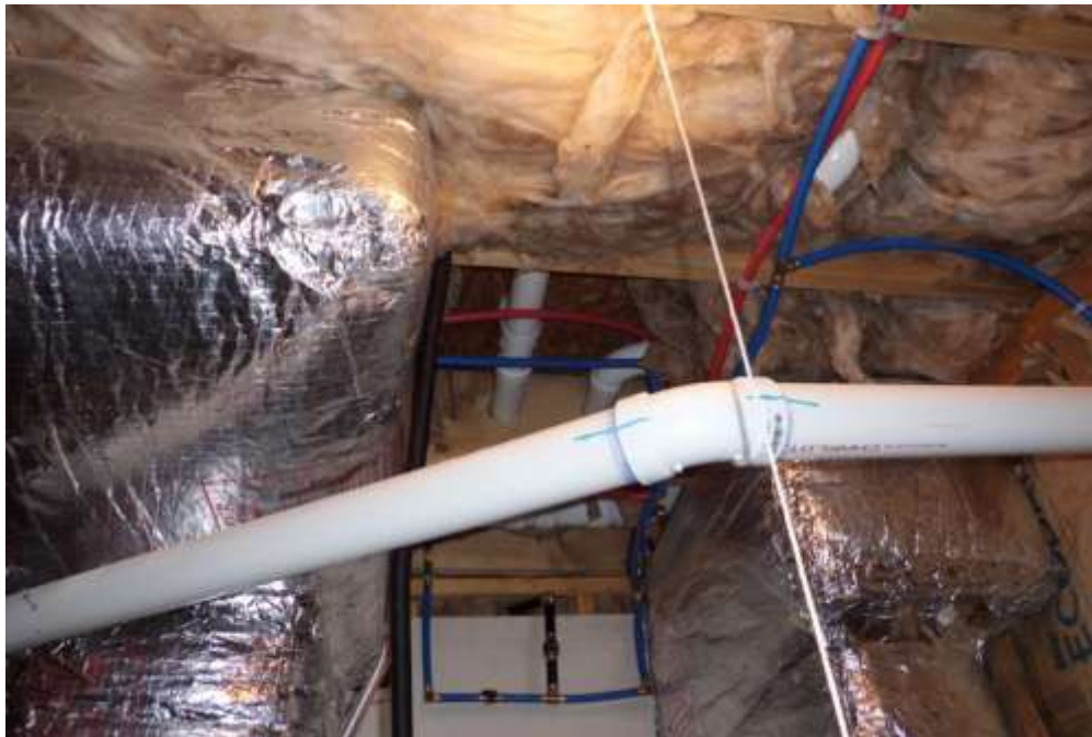
Figure E-6: Gaps in Frame Floor Insulation and Uninsulated DHW Lines
