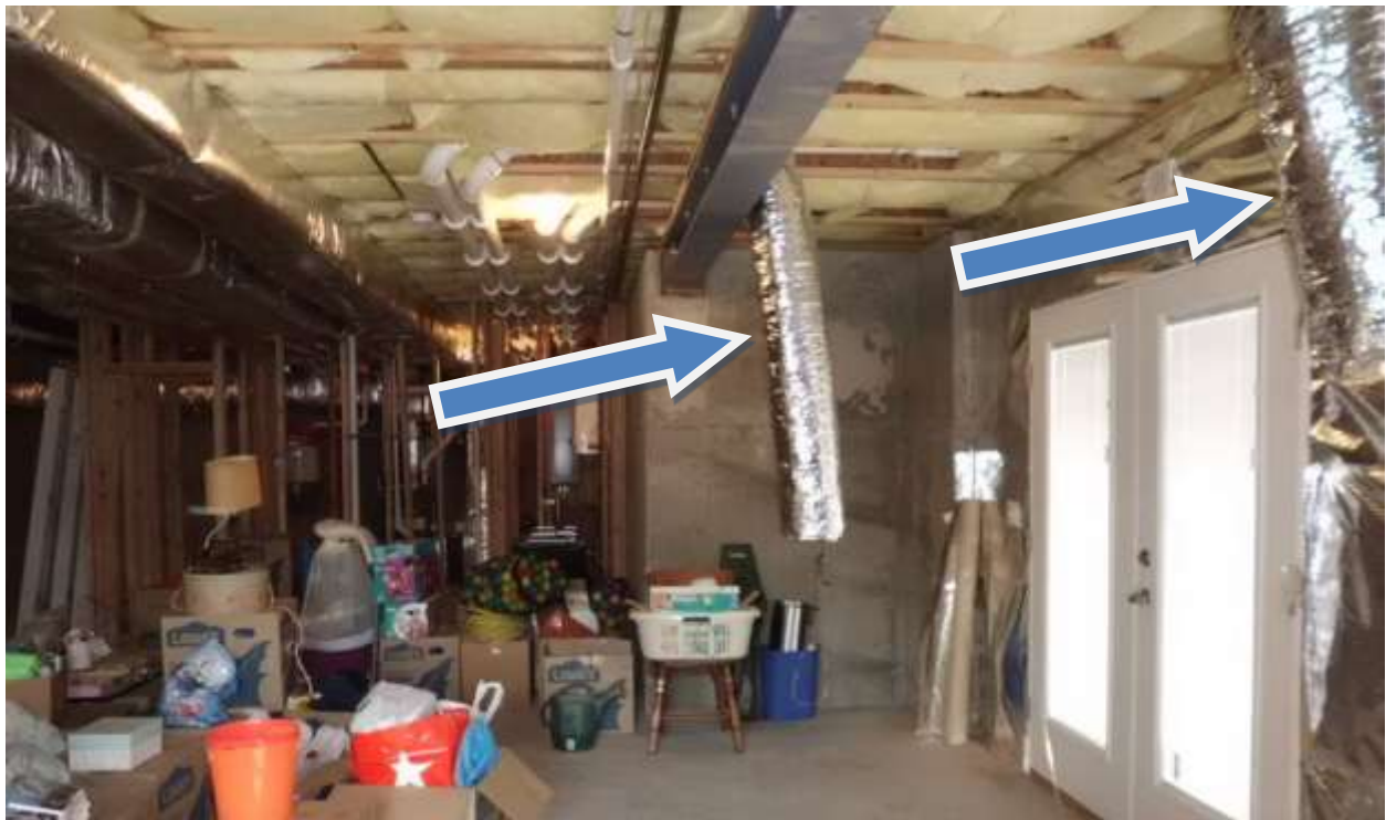
Figure E-17: Hanging Flexible Ducts Serving as Pressure Relief
