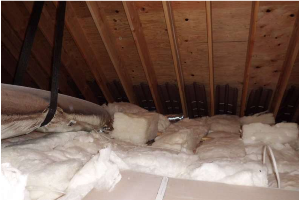
Figure E-10: Poorly Installed Fiberglass Batt Attic Insulation
