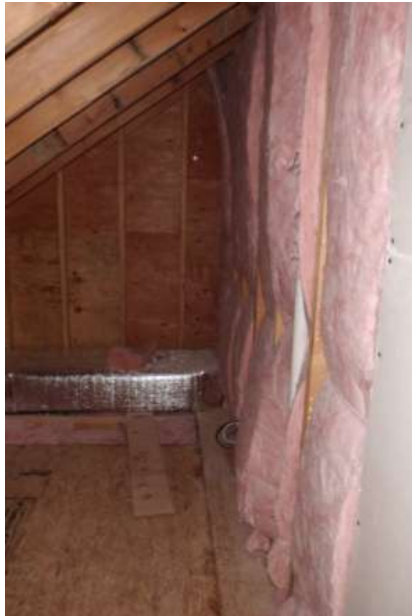
Figure E-9: Poorly Installed Fiberglass Wall Insulation
