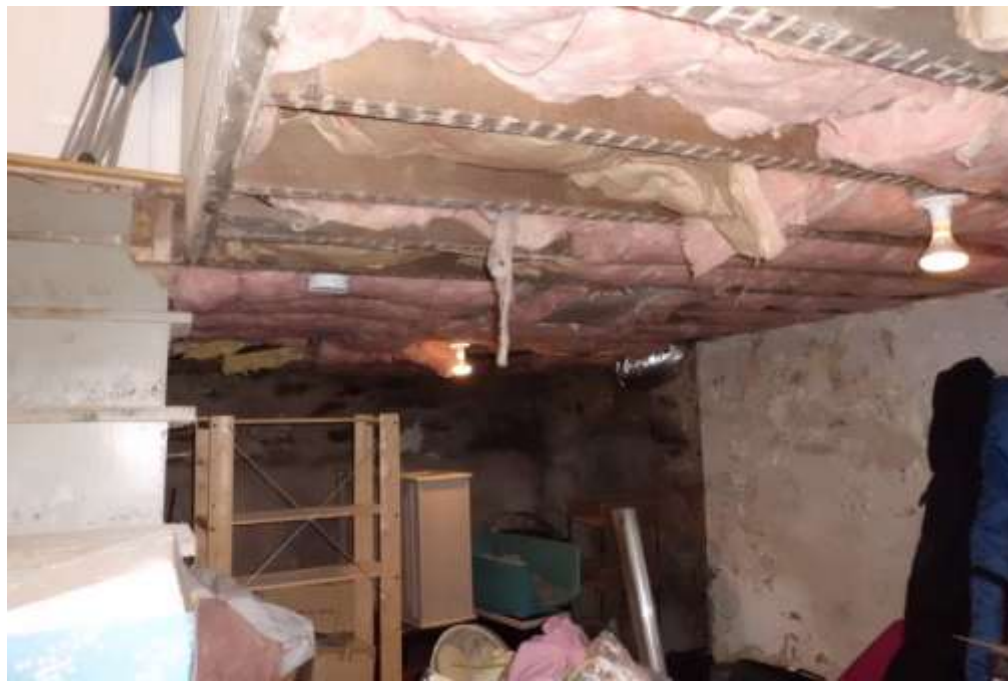
Figure E-4: Poorly Installed Frame Floor Insulation
