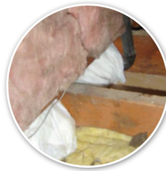
Figure 6. Air seal floor joist cavities under kneewalls by filling cavities with fiberglass batts that are rolled and stuffed in plastic bags (as shown here) or use rigid foam, Oriented Strand Board (OSB), or other air barrier board cut to fit and sealed at the edges with caulk.
