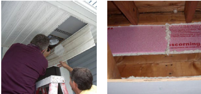
Figure 10. When researchers pulled back the porch ceiling, they found the wall board was missing so nothing was covering the insulation on this exterior wall. An air barrier of rigid foam board was put in place with spray foam (Image: Moriarta 2008).
