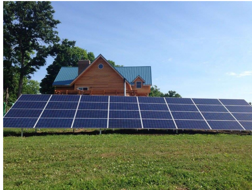
Small Ground-Mount Installations
